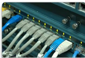
Cables must be connected correctly.
